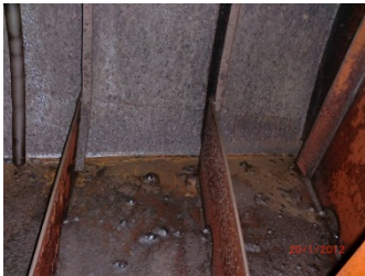
The bottom of a diesel tank, heavy microbial growth
