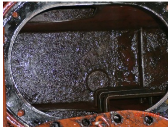
Diesel tank contaminated due to dirt, sludge and water
